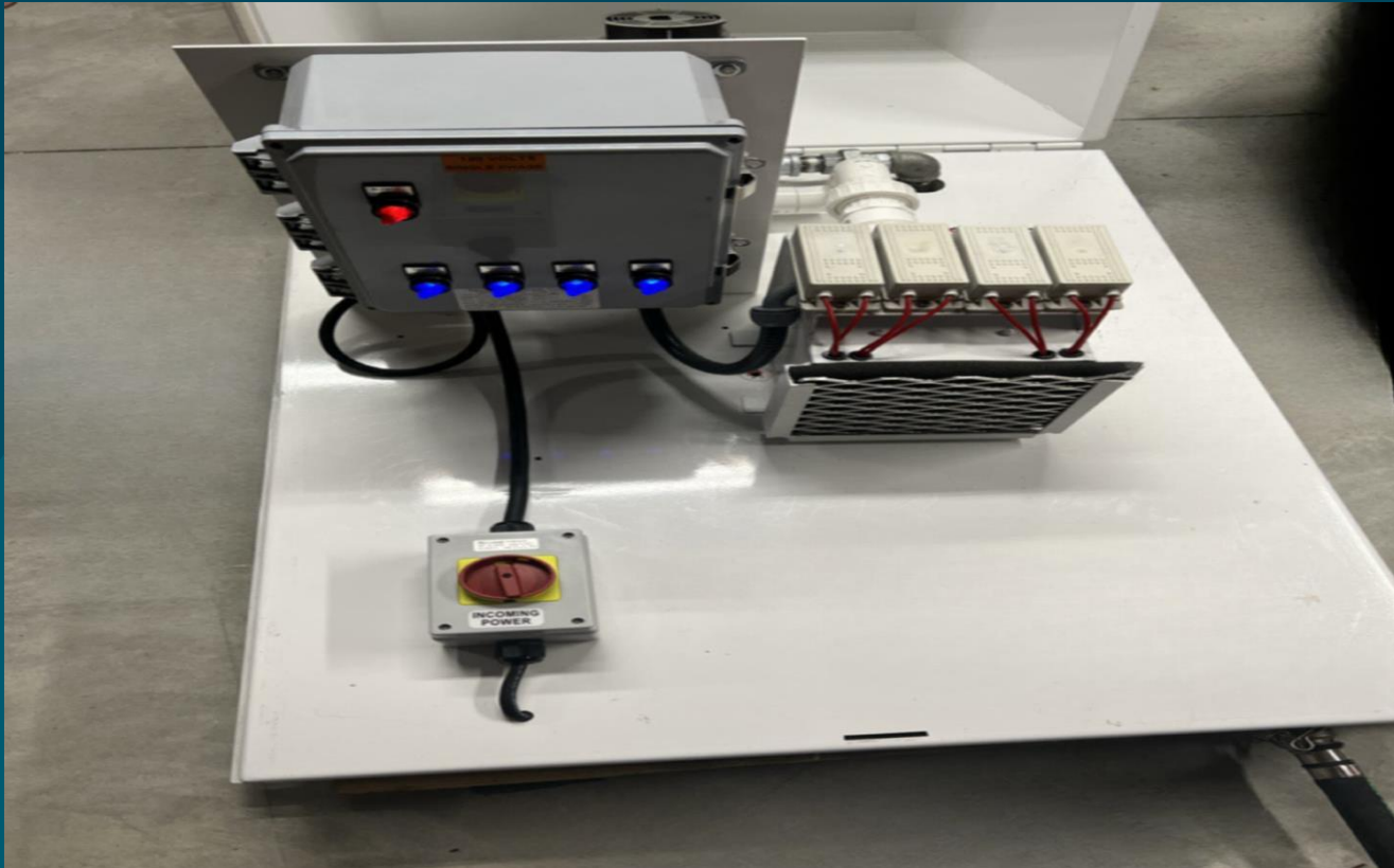
Picture: Demo Blower and O3 manifold
